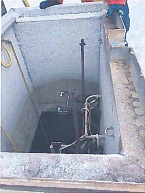
Dosing Chamber – Discharge Control Valve Stems (not operable)
